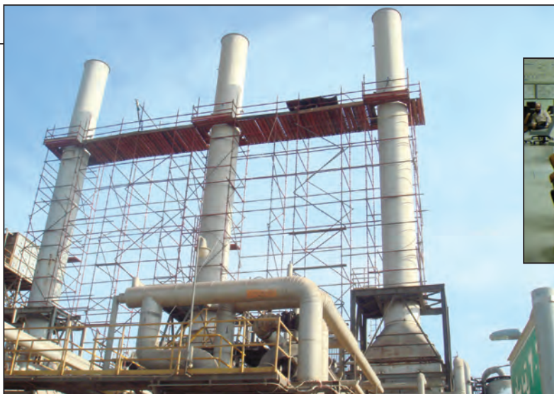
FIGURE 2. PEMS was implemented on the boiler stacks at Arrazi, three of which are shown here
